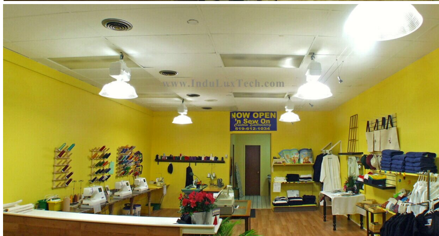
TOP: RETAIL STORE BEFORE UPGRADING TO INDUCTION LIGHTING BOTTOM: MAGNETIC INDUCTION FIXTURES INSTALLED IN THE RETAIL STORE
