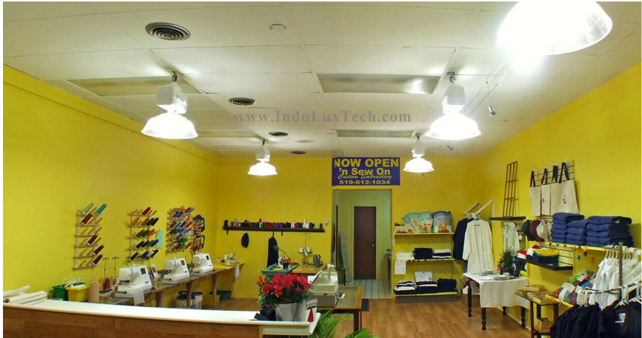
AFTER THE UPGRADE: A VIEW OF THE STORE WHERE 5 OF THE INDUCTION LOW-BAY FIXTURES ARE VISIBLE. NOTE THAT THE LIGHT DISTRIBUTION IS NOW MORE EVEN AND THE SPACE IS MUCH BRIGHTER.
