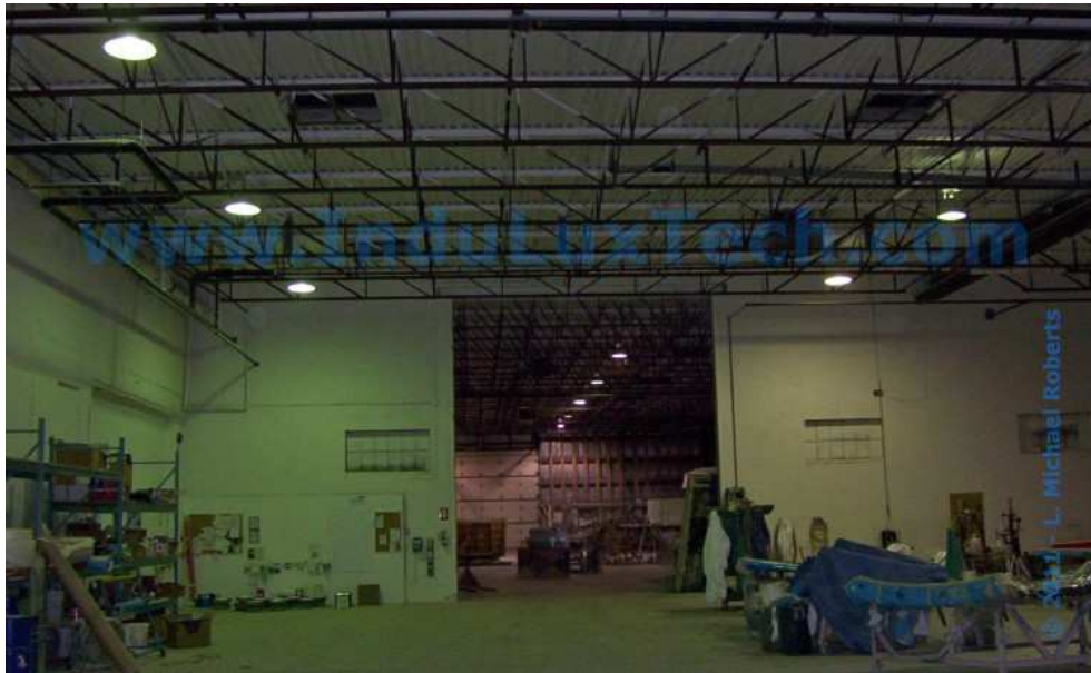
BEFORE: THE PRE-PRODUCTION AREA WHERE MATERIALS TO BE LAMINATED ARE CUT AND MEASURED (WORK TABLES AND BENCHES HAVE BEEN REMOVED TO FACILITATE A LIFT TO REACH THE LIGHTS). FIVE OF THE MERCURY VAPOUR HIGHBAY LIGHTS THAT WERE REPLACED CAN BE SEEN IN THIS PHOTO.
