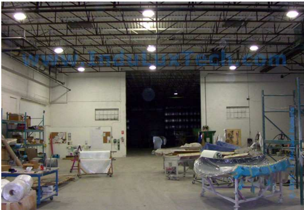
AFTER: THE COMPOSITES PRE-PRODUCTION AREA WHERE MATERIALS ARE CUT AND MEASURED IS SHOWN AFTER UPGRADING THE FACILITY TO INDUCTION LAMP HIGHBAYS. NINE OF THE INDUCTION LAMP HIGHBAY LIGHT FIXTURES AND ONE OF THE SECURITY LIGHT FIXTURES CAN BE SEEN IN THIS PHOTO.
